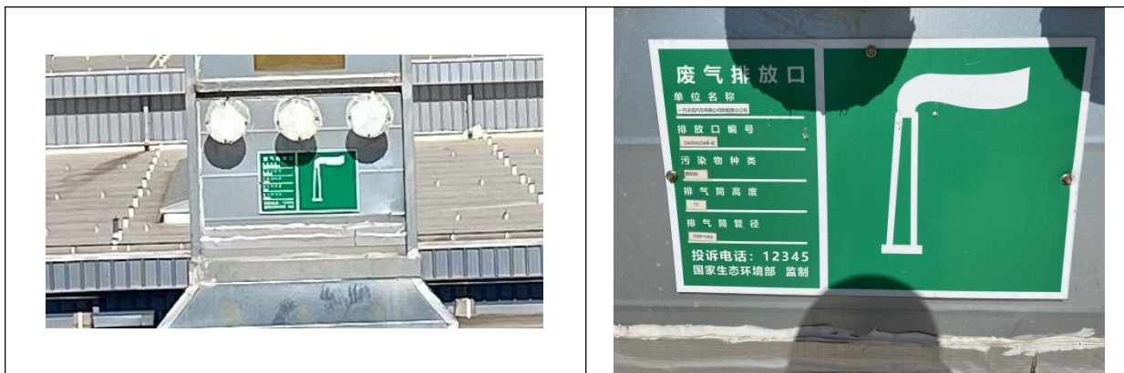
焊装车间小部件焊接排气筒 GW4-4 采样口
