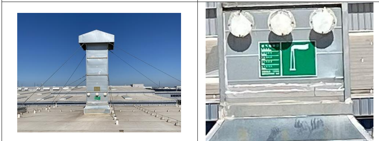
焊装车间小部件焊接排气筒 GW4-5
